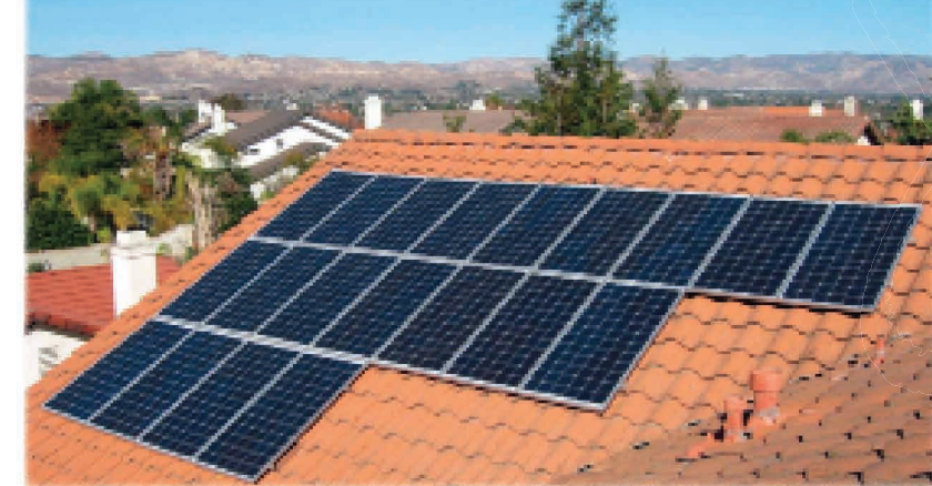
Solar electricity requires no moving parts, substantially decreasing maintenance requirements and increasing reliability and long equipment life.
